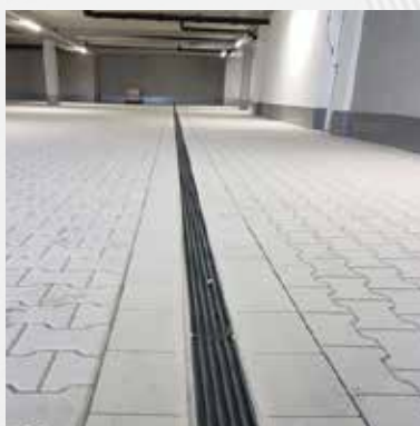
AquaStop in Pflaster
