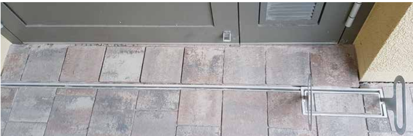
Entrance: Slot drain with catch basin and inspection cap, two keys
