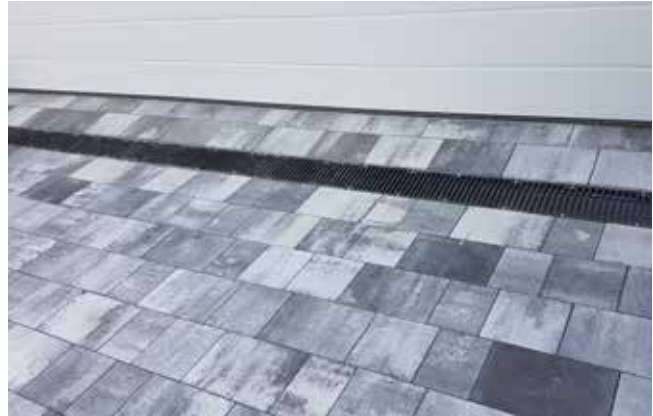
Garage doorway: 150V line with cast iron grating
