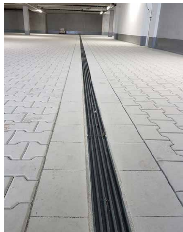
AquaStop in Pflaster
