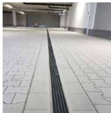
AquaStop in Pflaster
